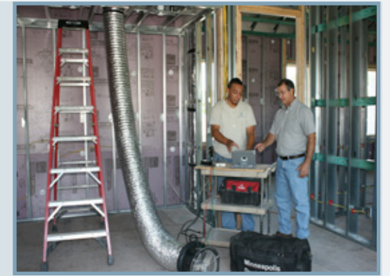
Edgar Garcia working with Building Science Director, Harold Robair, testing the A/C duct work
